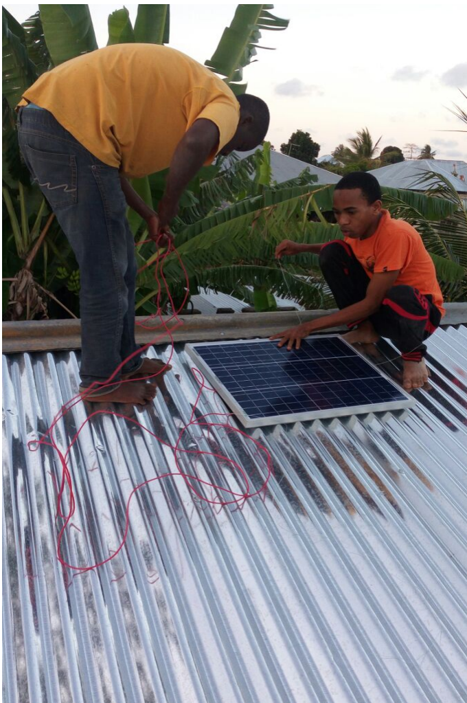
Tanzanian installation crew
