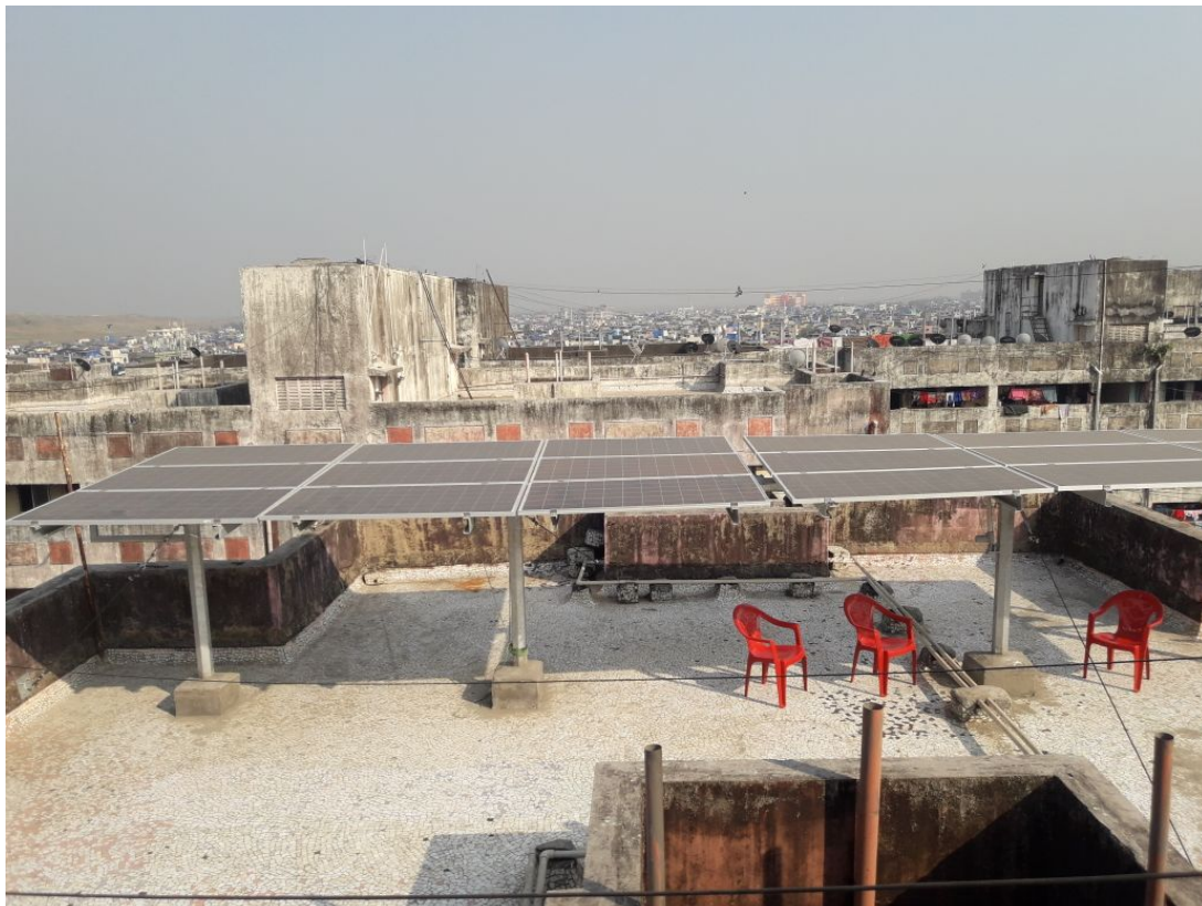
Mumbai rooftop PVs
