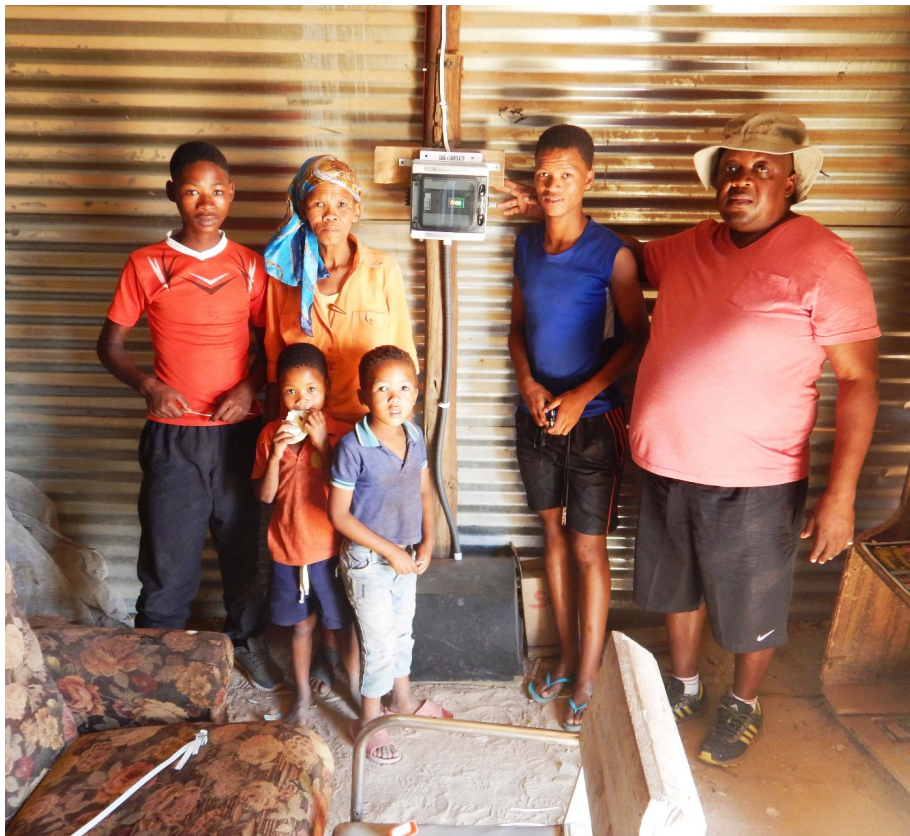
Newly installed household, South Africa
