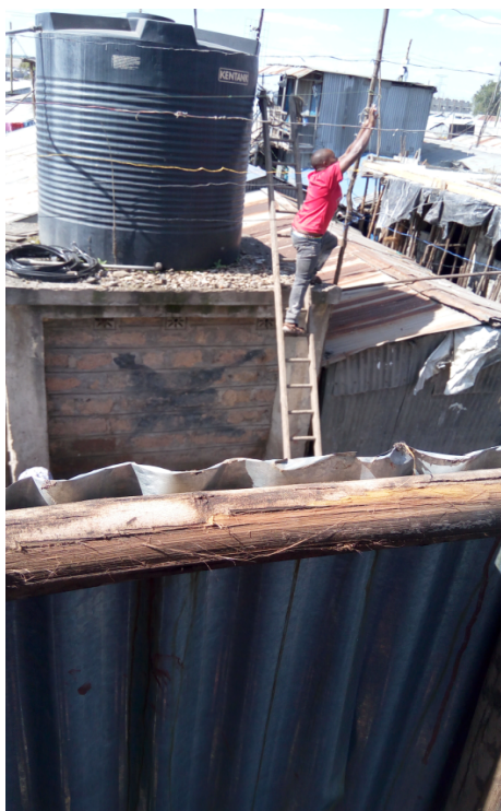
Informal electricity service, Nairobi
